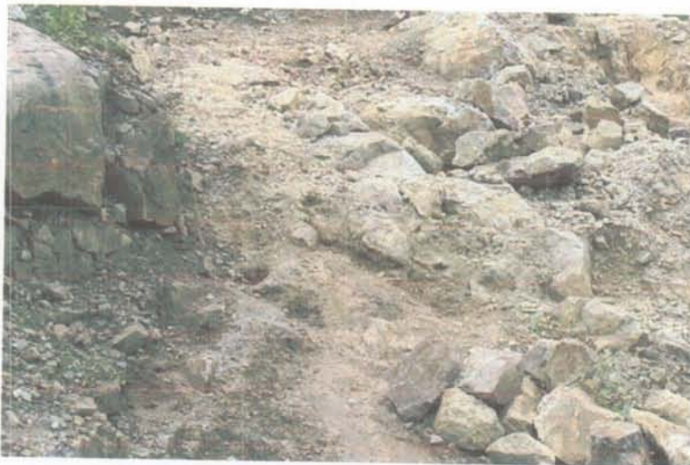
Photo 2: Looking west along work area. Bouldery till has been removed; initial wash-down of area performed. The large vein described above has just become visible in the lower left corner of the photo.
