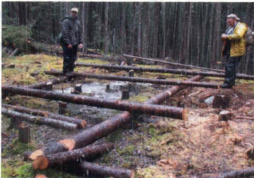
Figure 4. Drill site Can-08-17. Log frame used to support the Hydracore Gopher drill.
