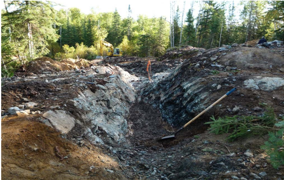
Figure 5: Excavation at Flint Rock showing in vicinity of old blast trench, looking east.
