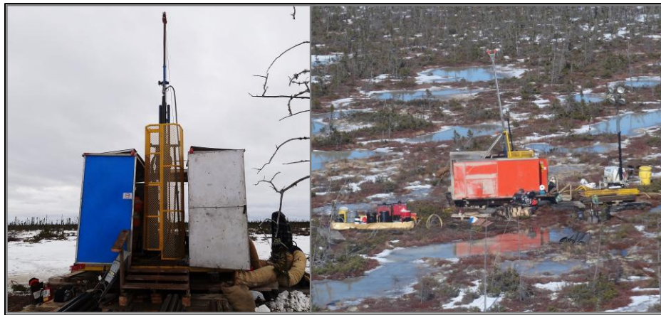
Figure 10. The Hydracore 2000 (left), showing the full cage guard, and the Zinex A5 (right) showing a common set-up of rig equipment
