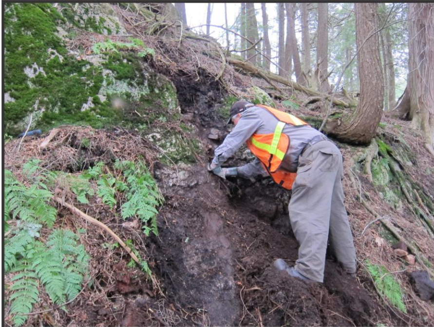
Figure 4; Photo showing fissure early on day one.
