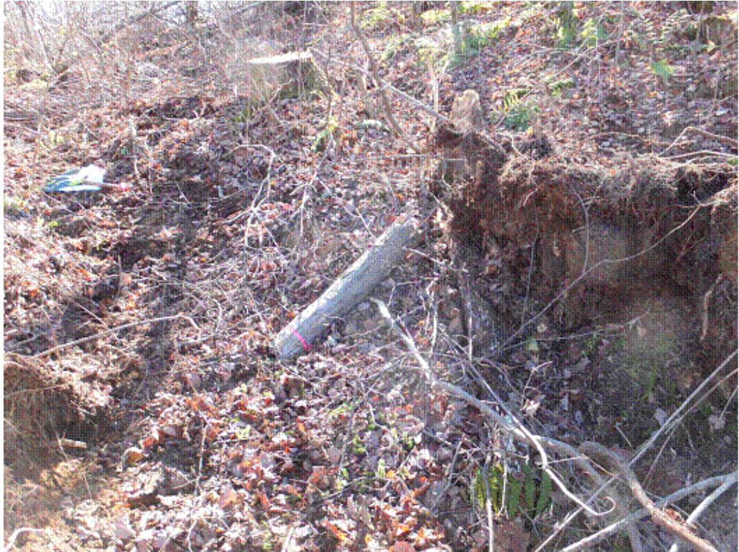
Photo Stump post damaged by forestry operations
