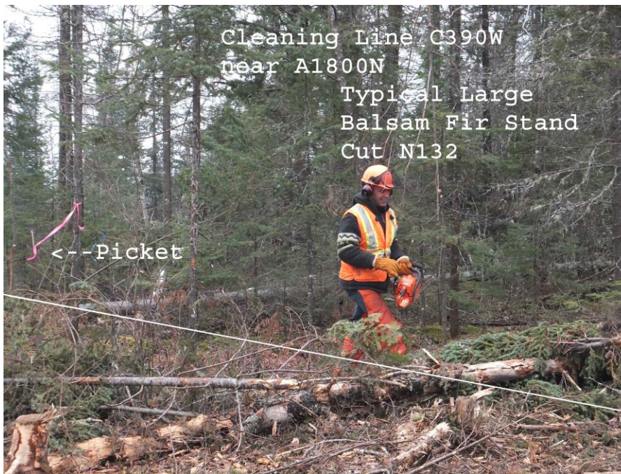
Nov 7, 2013, 2:10pm) Above photo: Glenn McBride's cutter clearing line in close proximity to A1800N.
