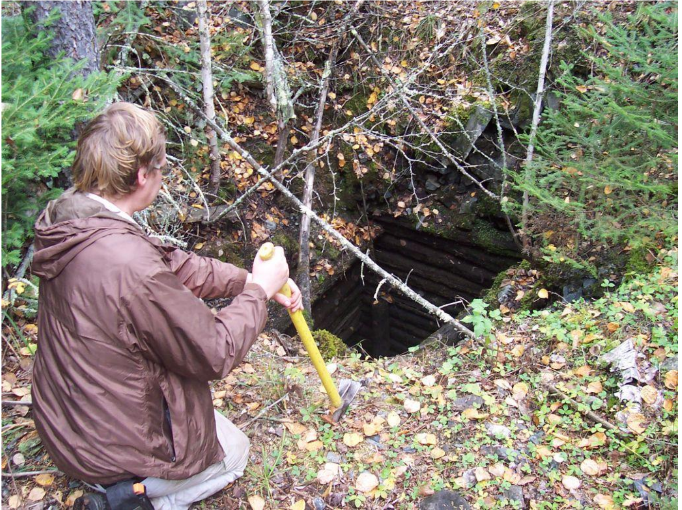
Photo 5. Looking northeast at Robert Hood looking down timber-cribbed open shaft at 570E/415N.
