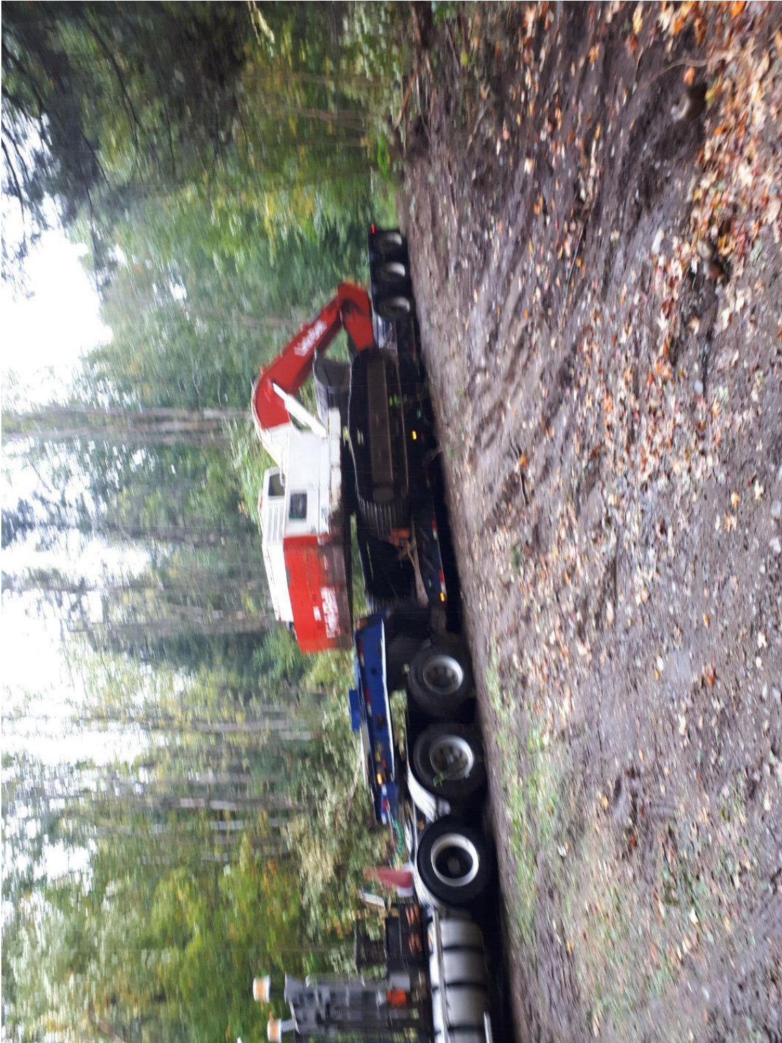
Photo of mobilizing LS-4300 Linkbelt excavator on site June 10, 2019 and off site on July 15, 2019.
