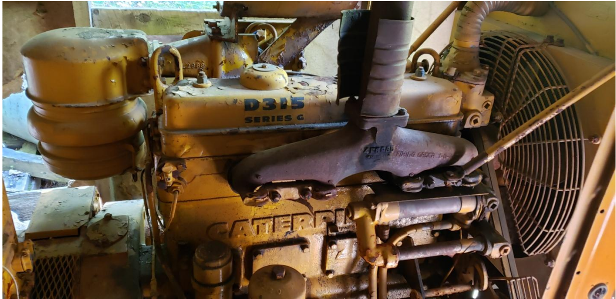
Generator to run the operation.
