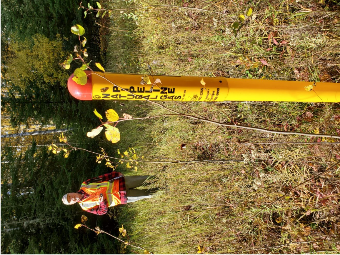
Figure 10 Gas Line on Claim 557534
