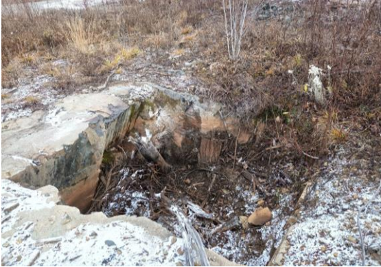
Figure 4: Photo of shaft, looking North. Note west side of shaft is broken to the N-S joint set of the diabase. A ten foot pole probed through floating woody debris could not reach bottom of shaft.
