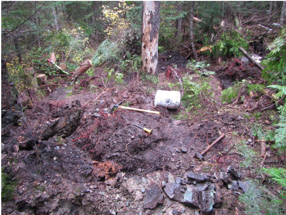
Looking north towards Little Esther Lake - Site preparation for October 2 nd to 4 th , 2021 manual trenching (minor brushing and removal of dead trees/brush)
