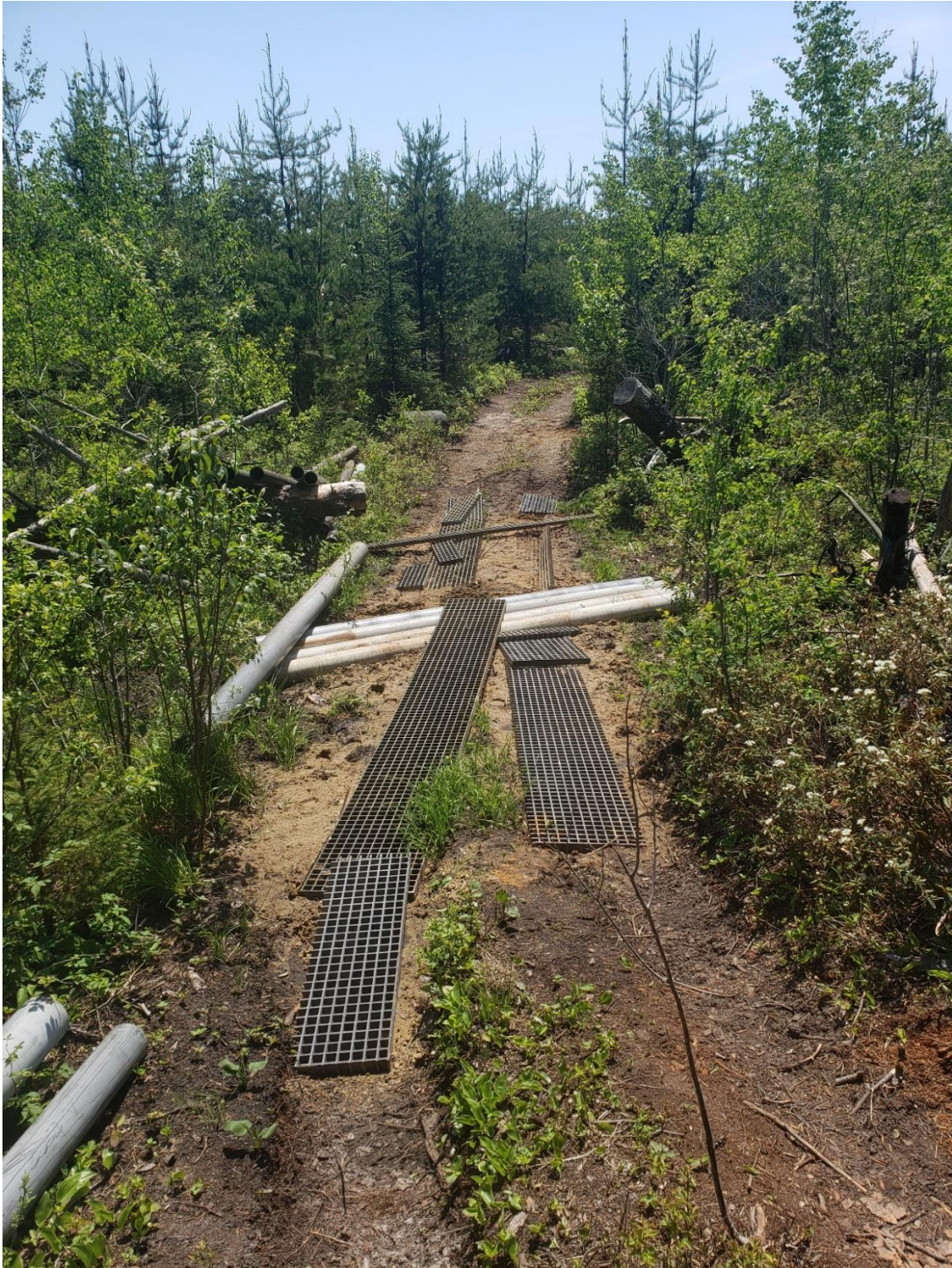
Figure 5. Shows initial site with fiberglass grating being initially and temporarily laid down to allow walking across the creek bed without sinking down.
