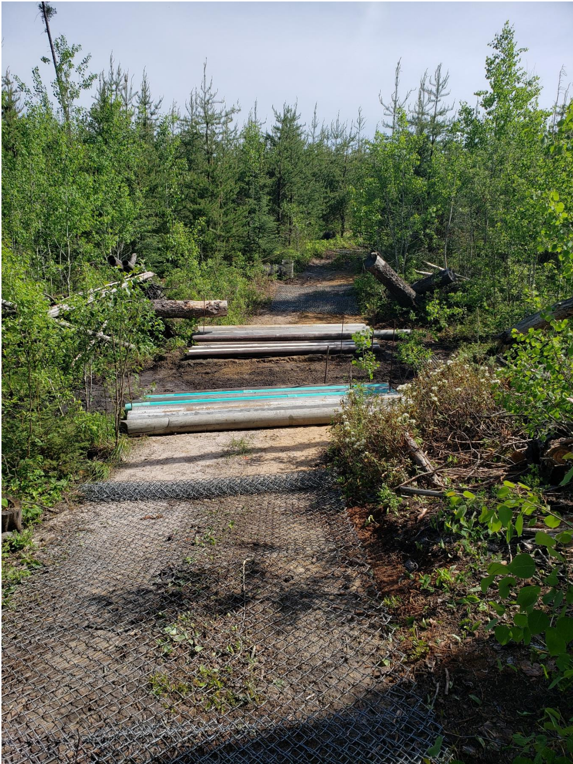
Figure 7. Shows some of pipes removed to allow exposing the bottom of the creek bed. Also shows the initial laying of the galvanized fence on both the North and South slopes of the creek to prevent erosion.
