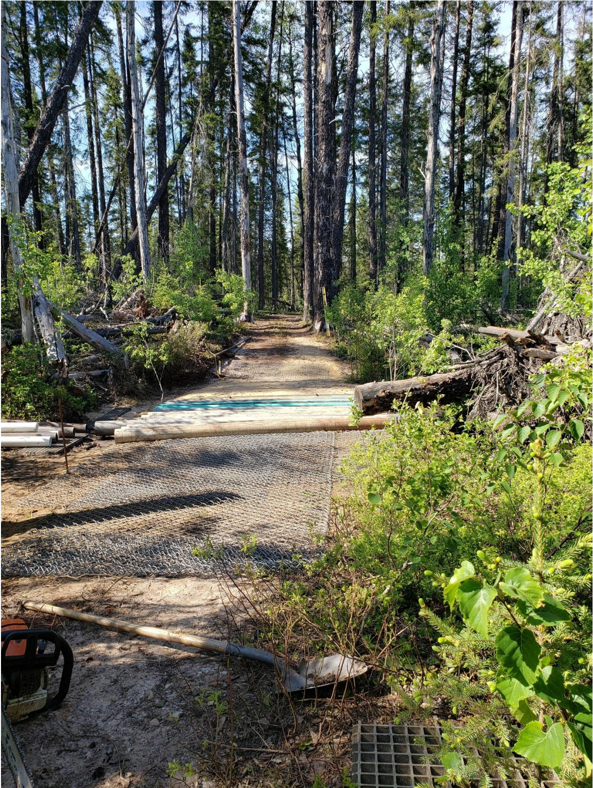
Figure 9. Shows the continued laying of the galvanized fence across the bed and slopes.
