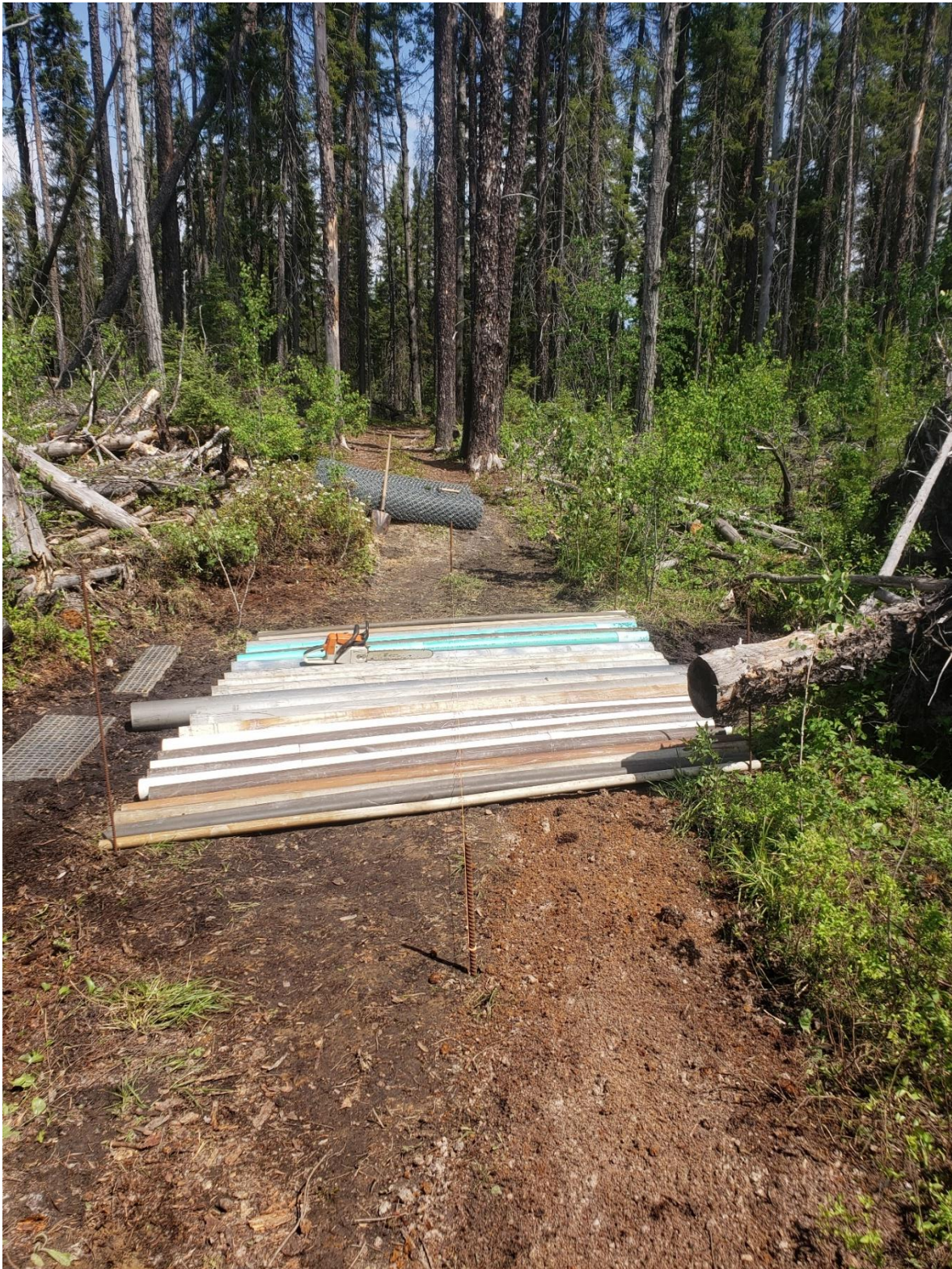
Figure 6. Shows initial and temporary laying of pipes longitudinally and in line with the natural flow of the creek (Westerly to Easterly flow). Pipes later removed to allow exposing the natural bottom of the creek bed.
