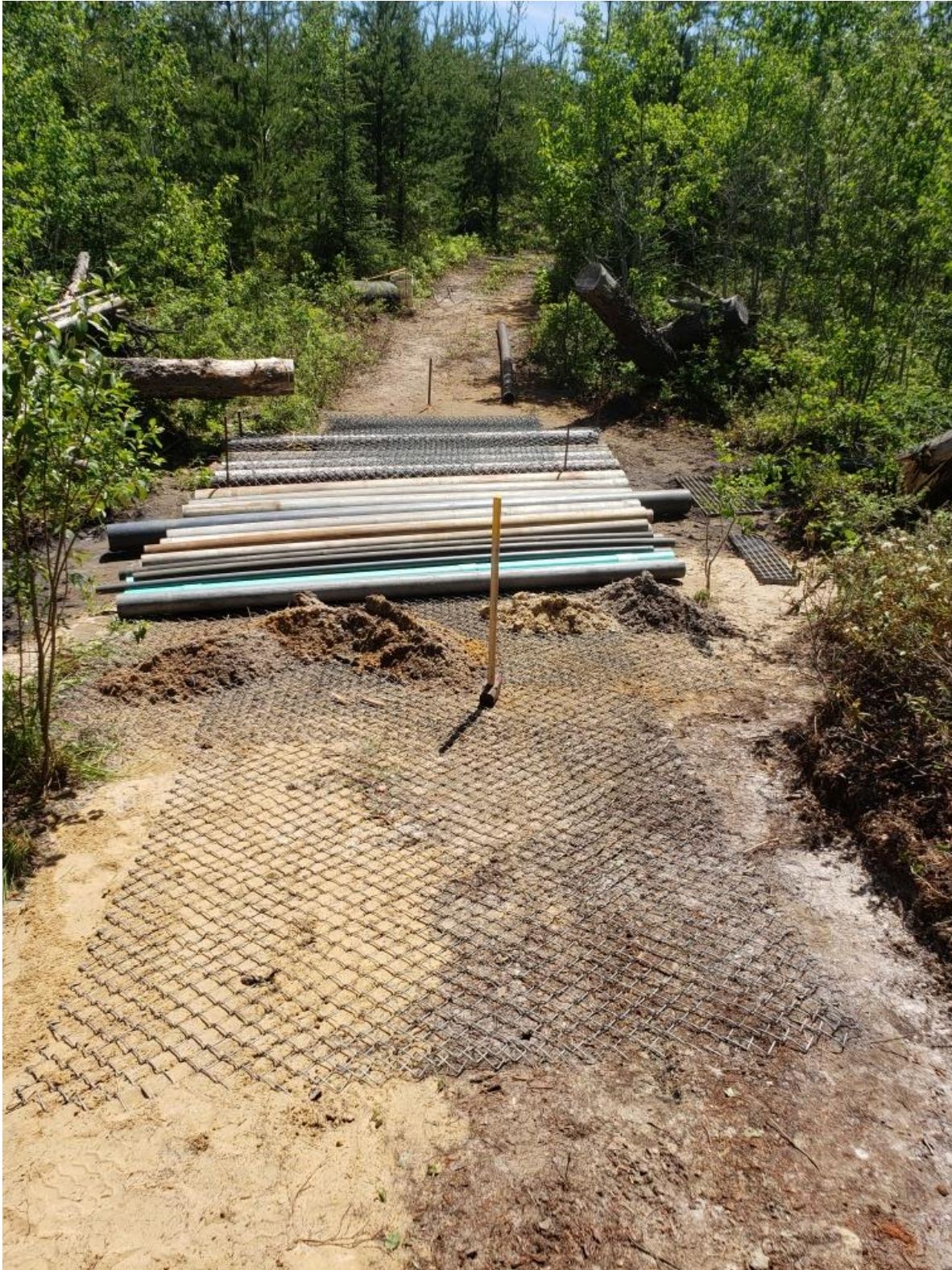
Figure 10. Shows the continued laying of the galvanized fence across the bed and slopes. Sand from a nearby sand pit was continuously added to the approach slopes.
