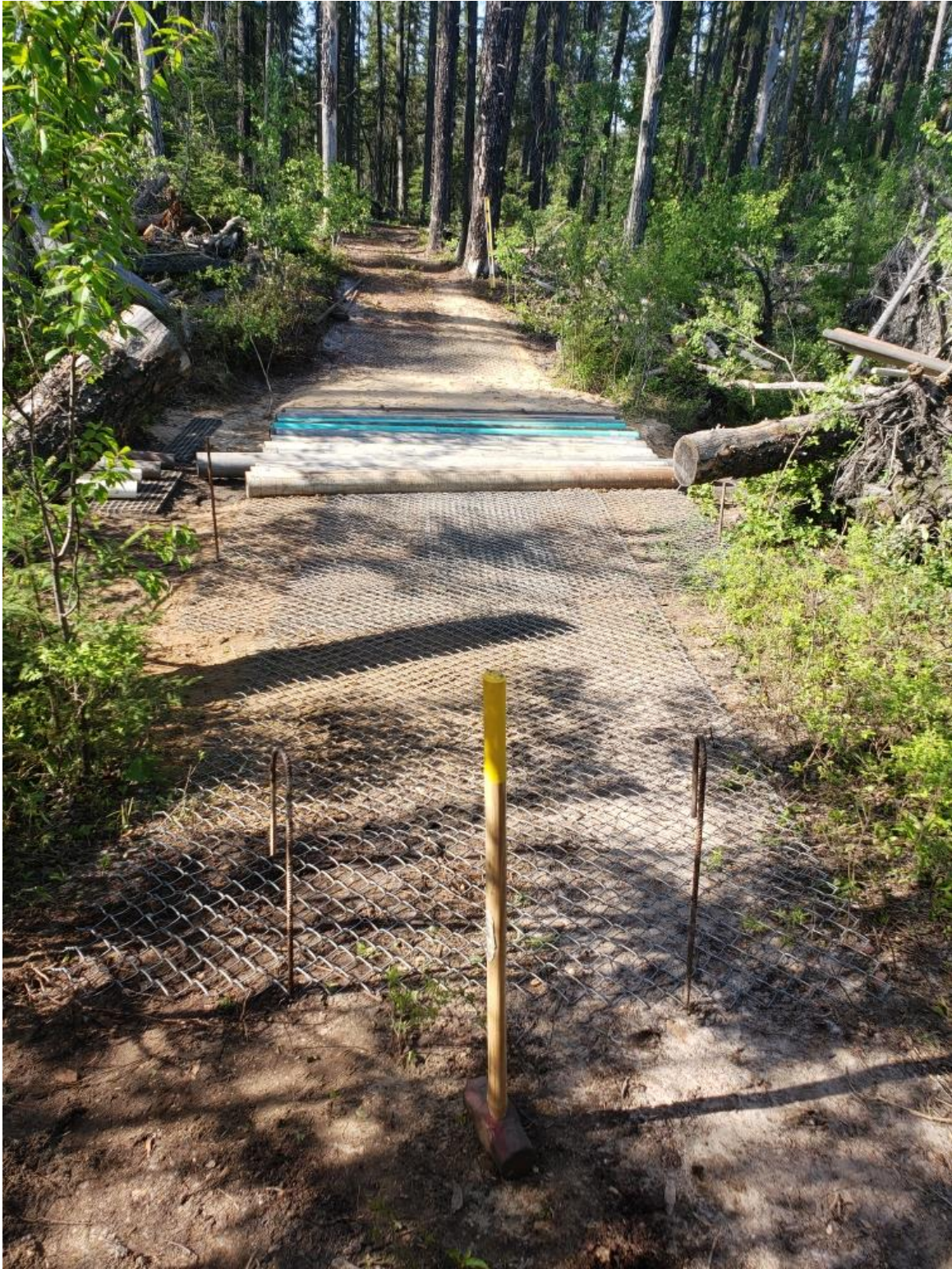
Figure 12. Shows the galvanized fence being secured down with 6' lengths of ½ inch rebar (already down 4' in picture).
