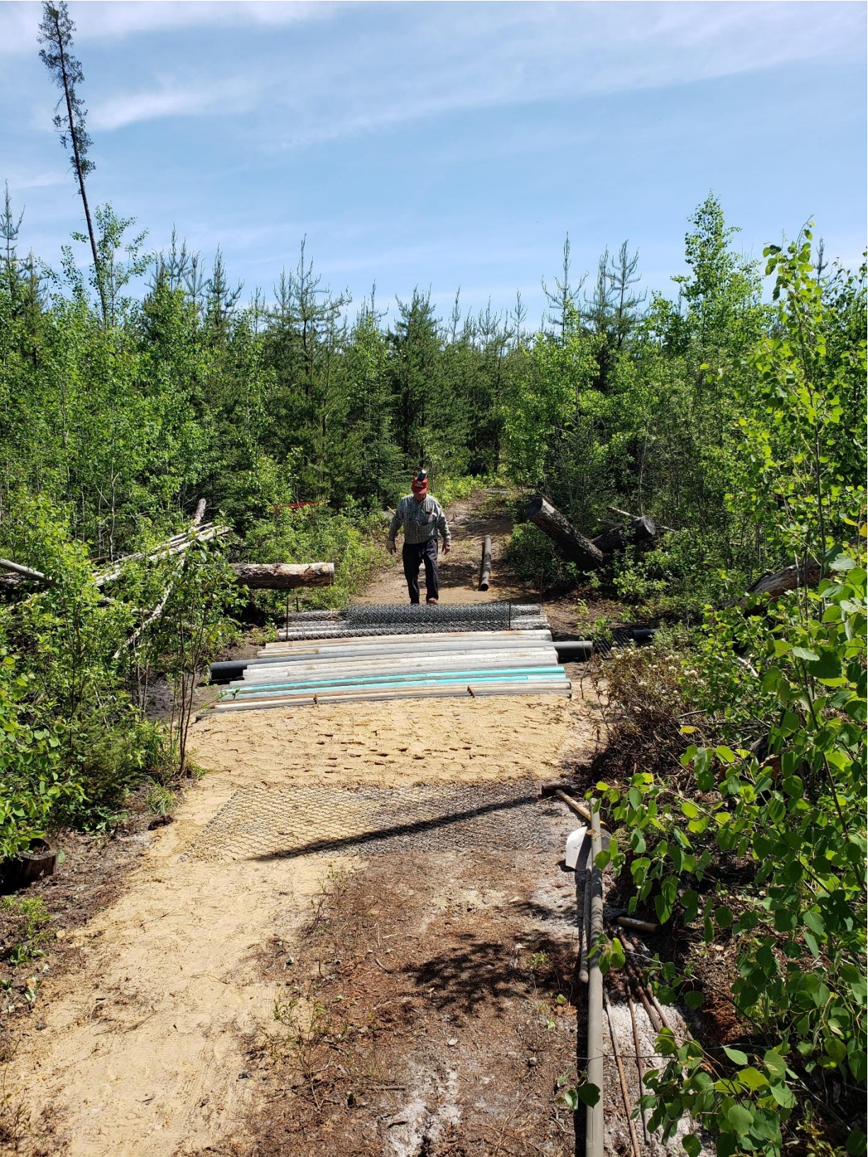
Figure 8. Shows the continued laying of the galvanized fence across the bed and slopes.
