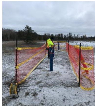
Groundwater Monitoring (three wells on tailings protected by snow fence)
