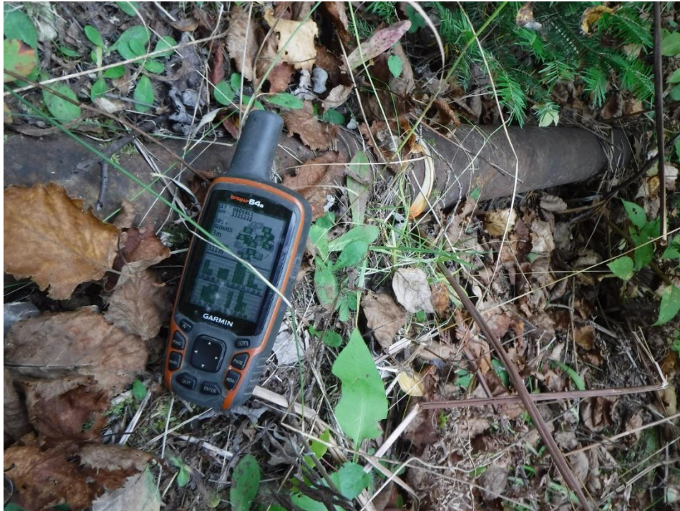
Figure 4: Broken Casing Located
