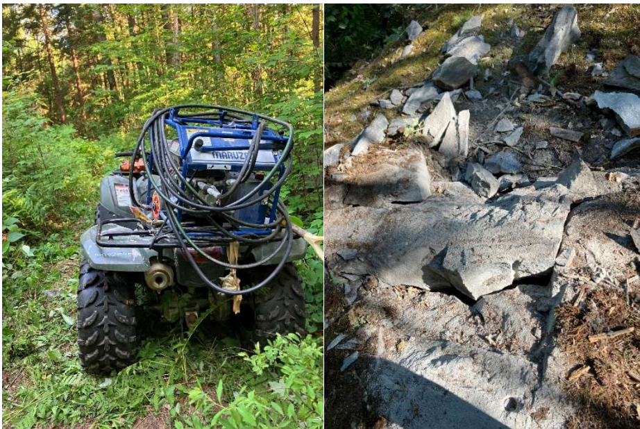
Figure #7 Small Scale Equipment all fit on ATV. Outcrop exposure with shallow blasting to expose rock
