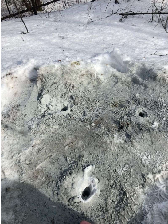
Figure #3 Drill holes completed on March 20, 2022 using rented Copco Drill I carried in on the snow.
