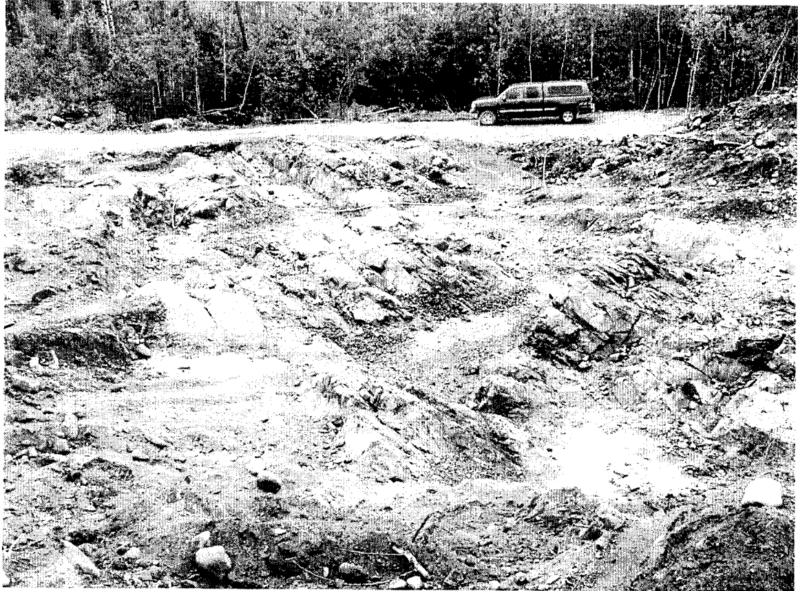
D65 showing – stripped area.
