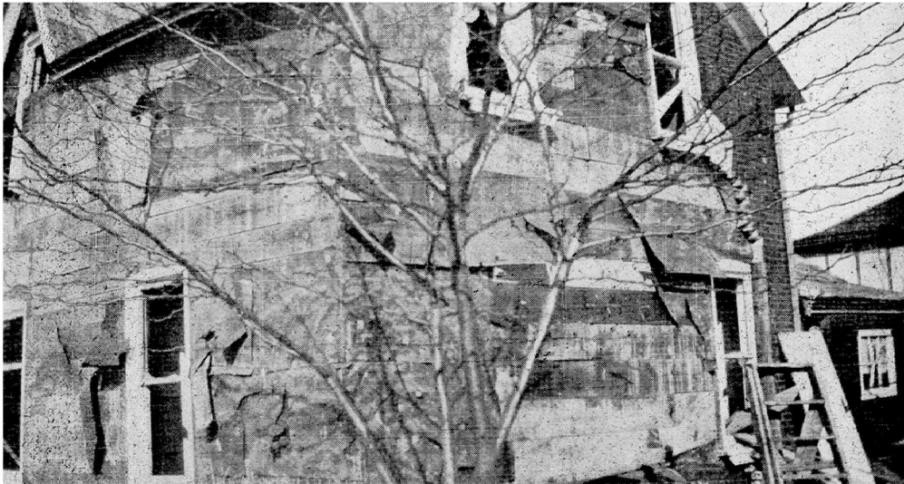
The photograph shows the results of an explosion of natural gas in the cellar of the home of Mr. D. M. Lee, on the outskirts of the city of Paris. A leakage of gas from an outside source found its way up a drain-pipe into the cellar, and a match ignited it. The house was practically a total wreck, as can be seen in the photograph; the brick veneer was completely demolished; fortunately there were no serious casualties.
