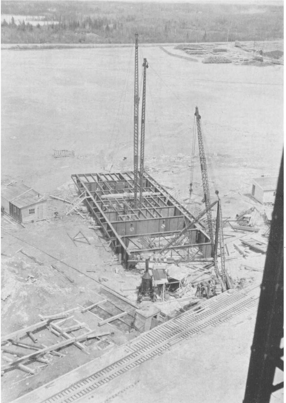
View from the water tower of Lake Shore Mines showing construction of the steel deck for the new No. 5 shaft.
