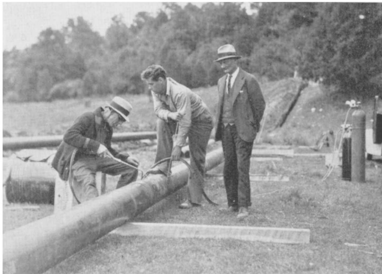
Welding the section of the pipe line to London that is to be laid under the Thames river.
