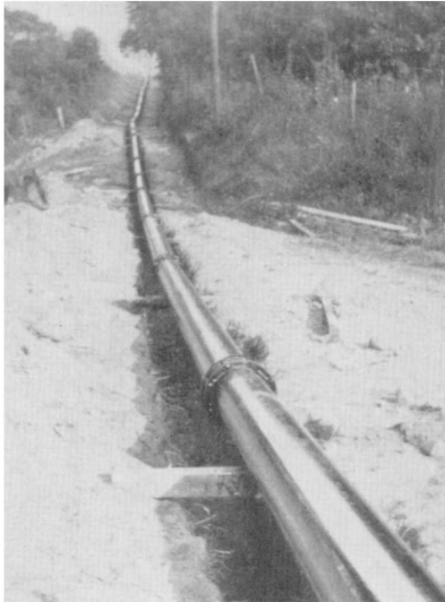
A section of the Union Gas Company's 10-inch pipe line from the Dawn gas field to London. This pipe has been coated with a rust-resisting material and is now ready to be lowered into the trench.
