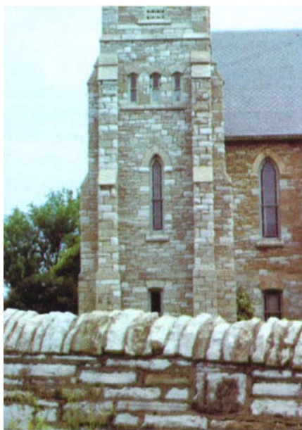
Photo 50 St. Peters church at Madoc, built in 1853, showing the use of local Black River limestone in the form of rock faced random ashlar.
